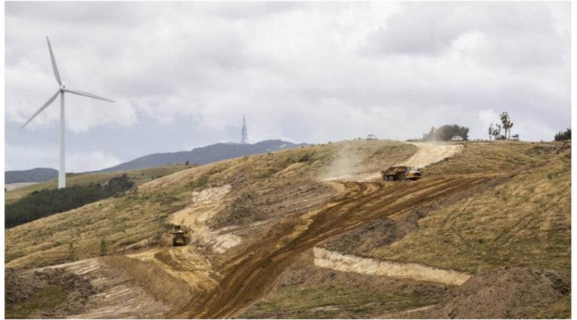
Earthworks are filling in a section of gully near Ashhurst where the new highway will run.
