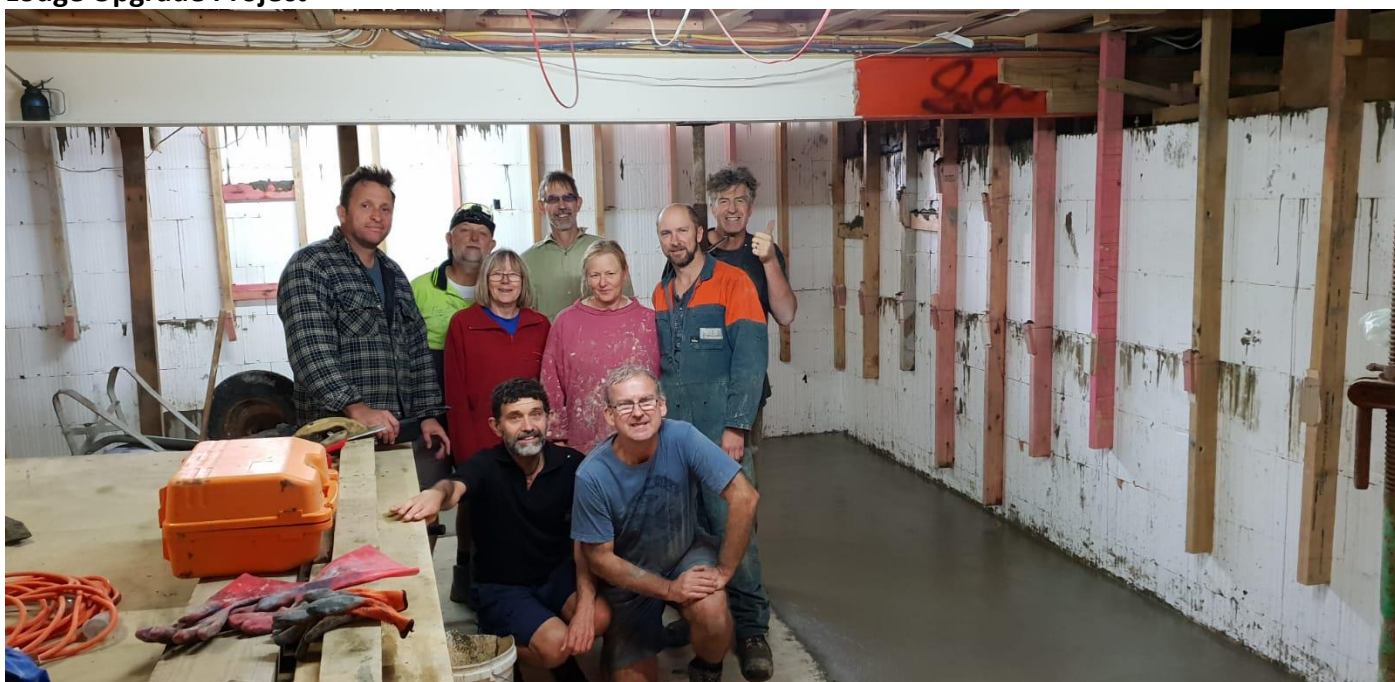
The final concreting crew, tired but happy, in the basement of the lodge beside the floor extension & surrounded by polystyrene blocks full of concrete.
