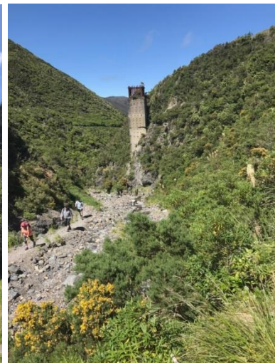
The Wrecked Bridge and Barrier
