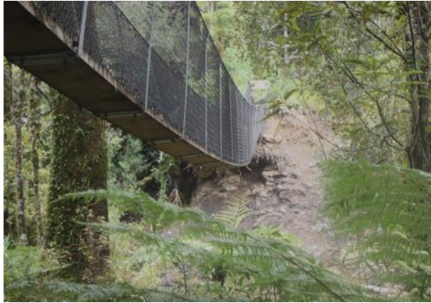
The undermined bridge
