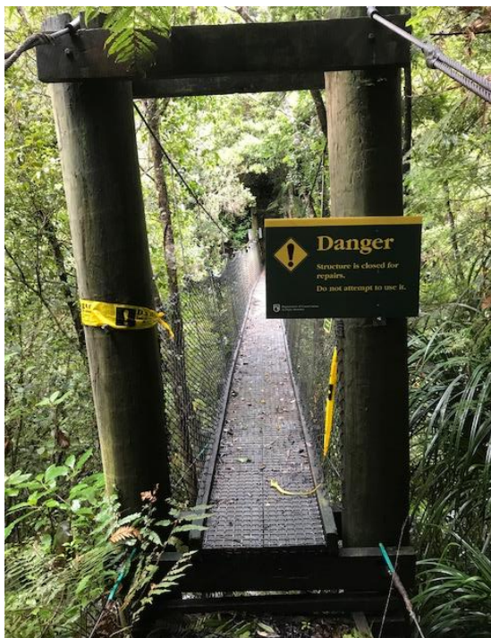
The 'unsafe' bridge
