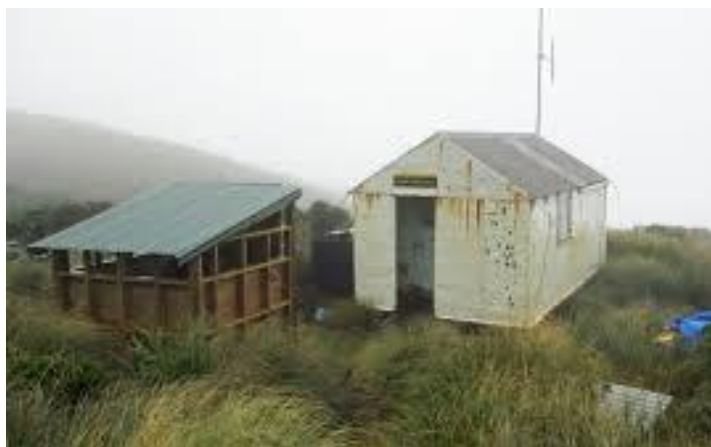
Cattle Ridge Hut looking very sad before work was done
