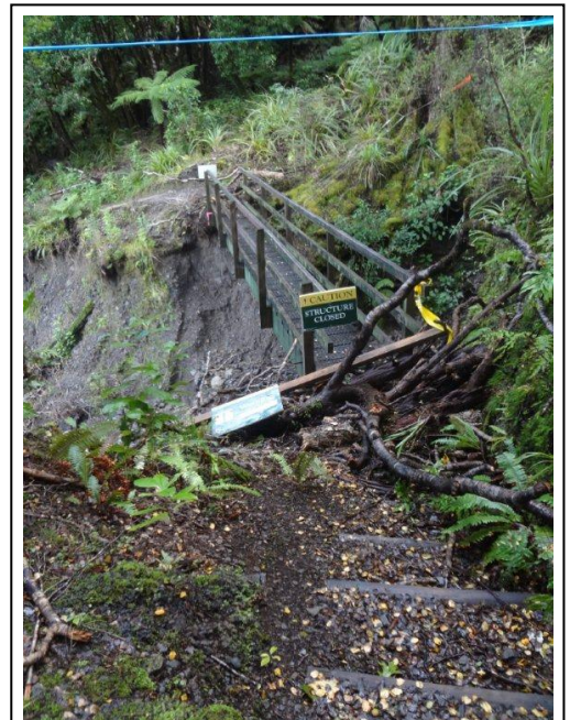
Washed out bridge
