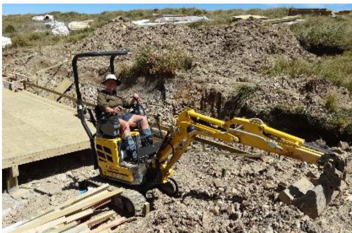
Jean doing some of the earthworks for the new Kime hut. See Tregear trip report on pg6. Image A.Match
