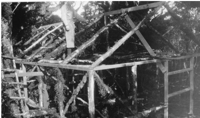
Building the first Te Matawai Hut. 6-13 Jun 1932. Image by Andrew Fuller, from the MTSC collection.
